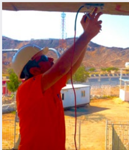
Fire Damage Assessment
