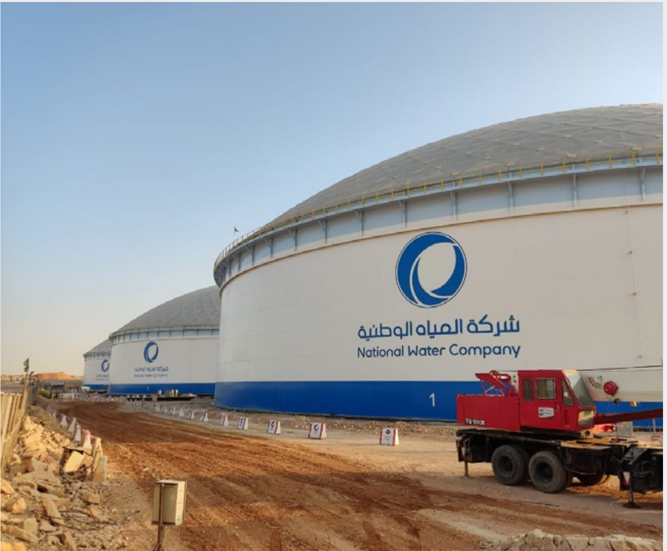
NWC Water tanks
