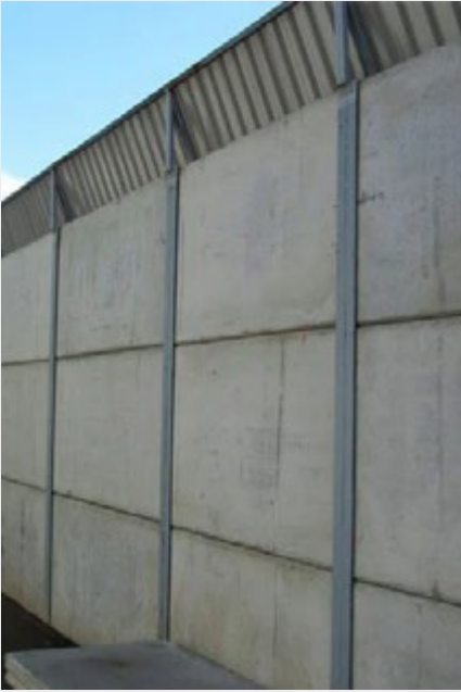
Hollow Core Boundary Wall
