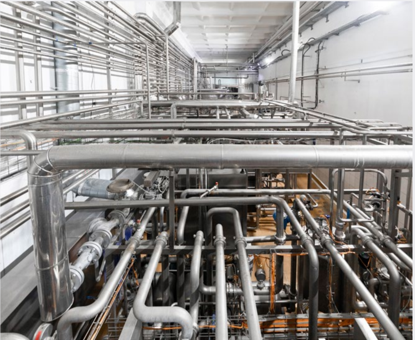
Plumbing & Piping Systems
