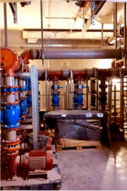
Plumbing & Piping Systems
